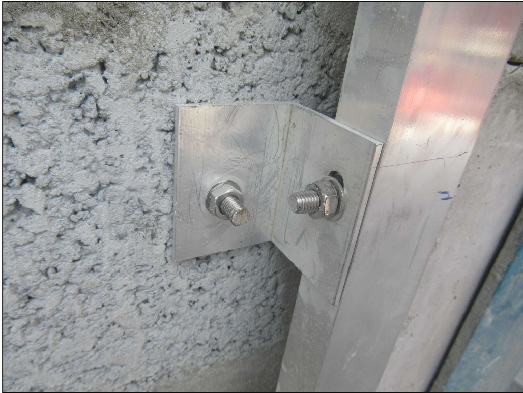
Picture 1: The runner fastened to the wall bracket which was in turn anchored to the block wall.
